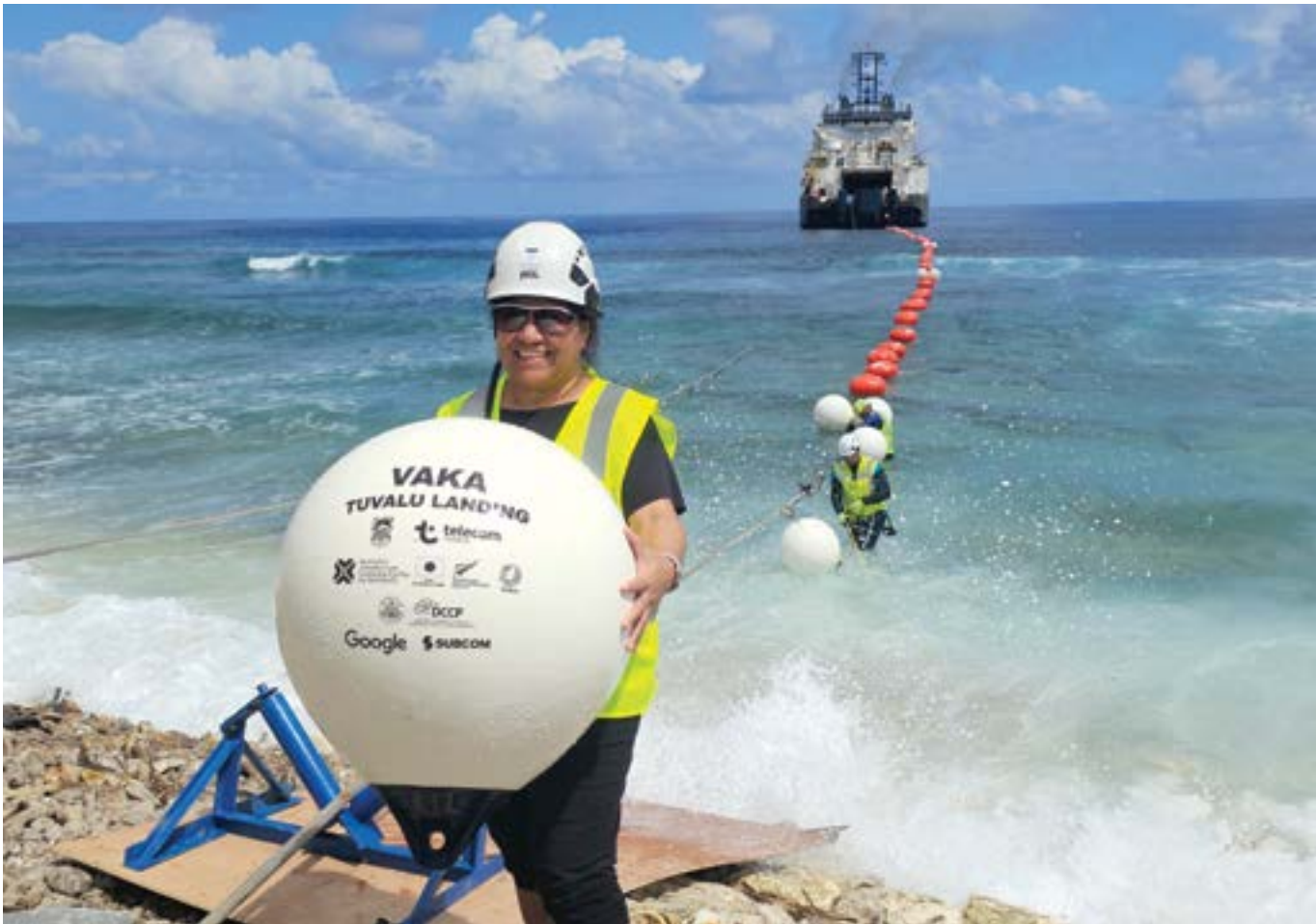
Image: Tuvalu Telecommunications Corporation CEO Tenanoia Simona at the Tuvalu Vaka Cable landing in Funafuti.
